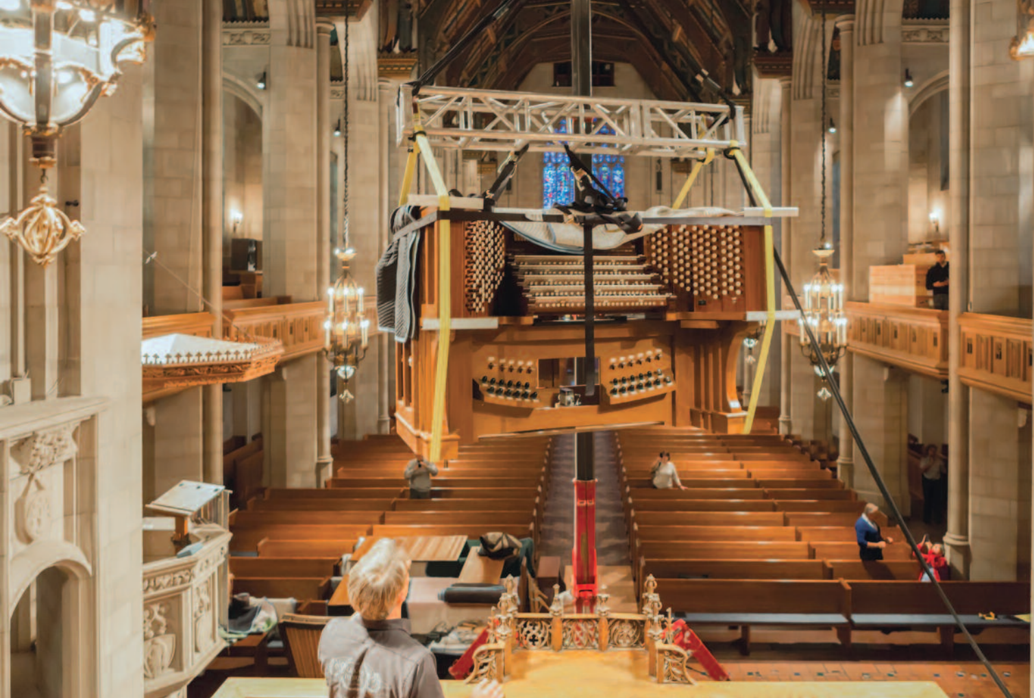
Above: Opus 71's five-manual console being hoisted into the choir loft; left: the Positiv casework
